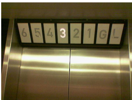
fig.7. Lift Floor Indicator.
